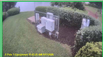
.5 Pole 1 Equipment 11:47:25 AM 9/17/2026
